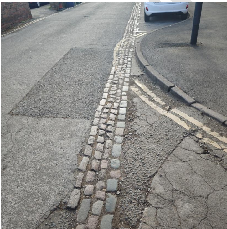
Figure 18: Unsympathetic and patchwork repairs to road surfaces
