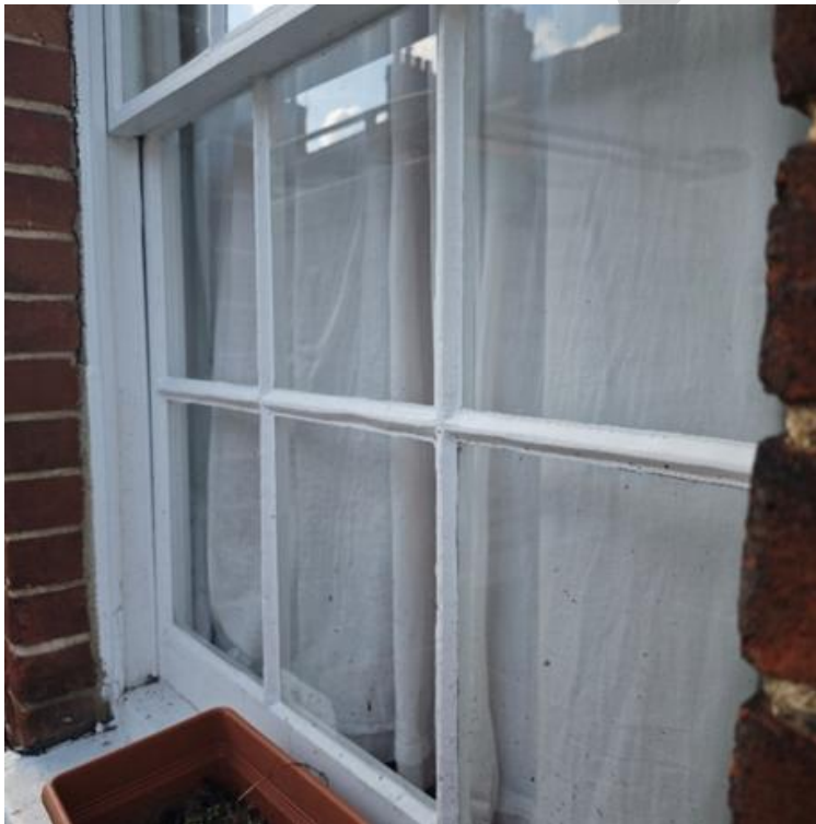
Figure 84: Original timber vs. Modern sympathetic replacement
