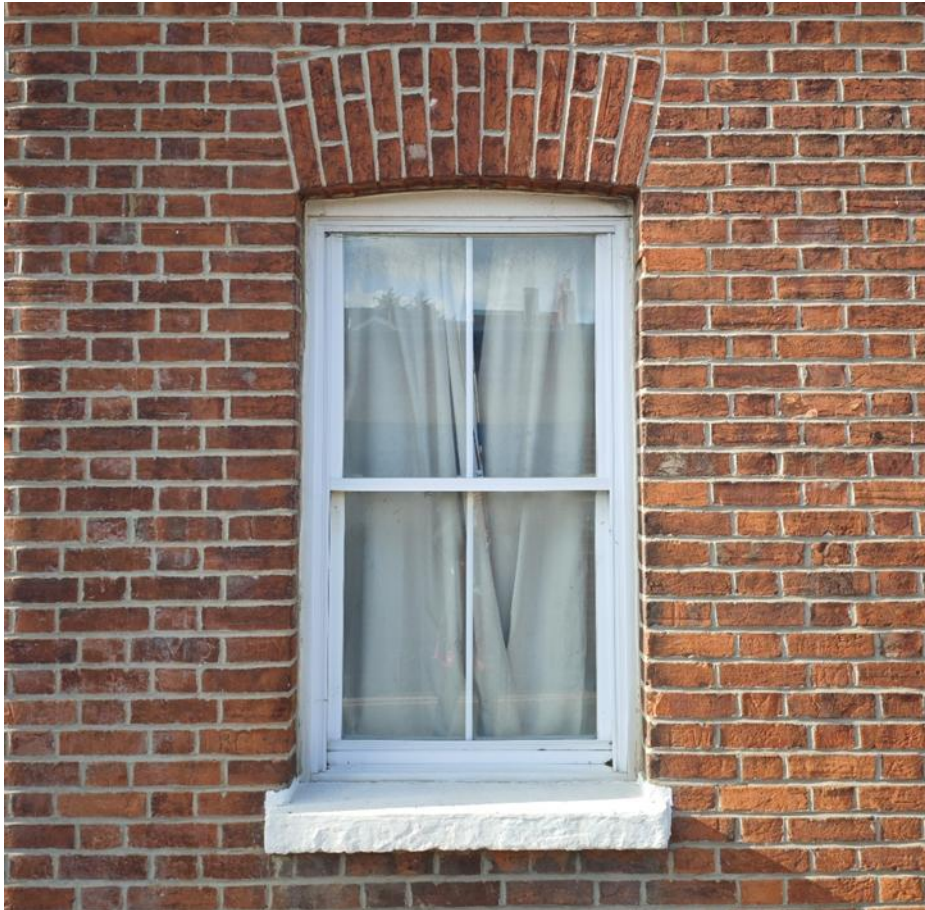
Figure 43: Some windows have been unsympathetically replaced with PVCu, and original 6-over-6 sash design has been lost
