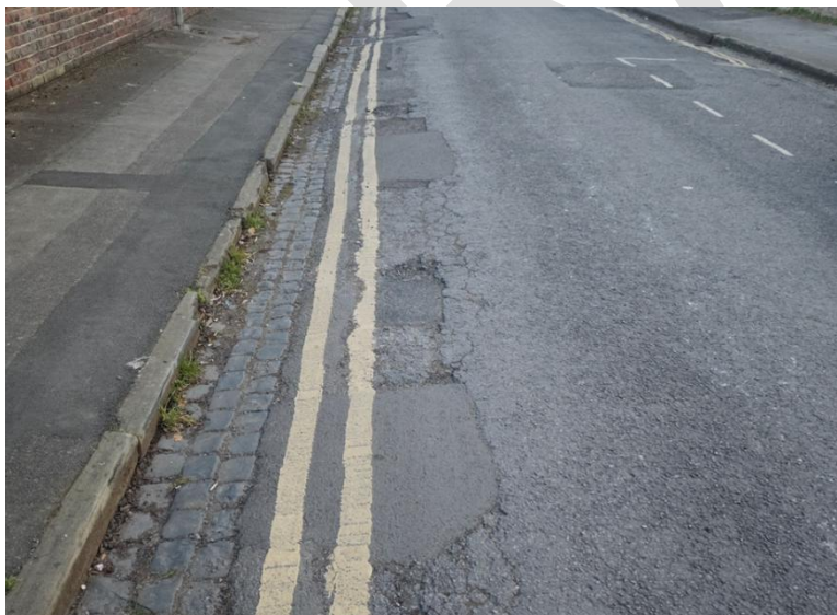
Figure 74: Road and Pavement surfaces in poor condition and inappropriate replacement of traditional stone kerbs with modern concrete which are liable to cracking and deterioration.
