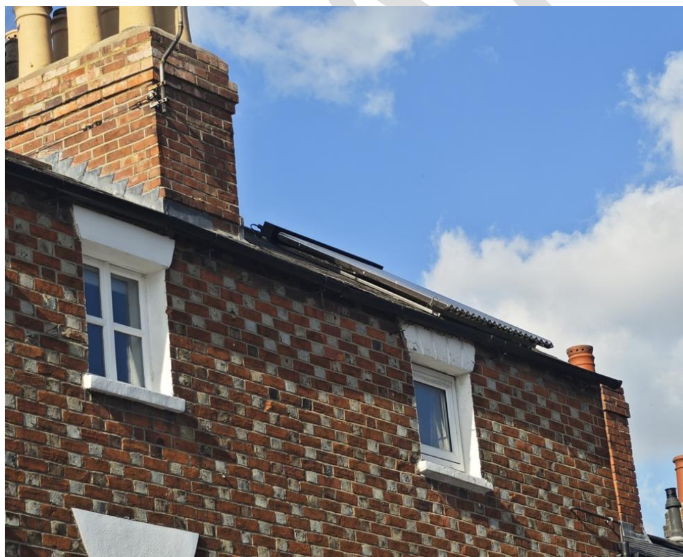
Figure 69: Original timber sash windows replaced with modern PVCu with thicker frames and trickle vents detracts from building's significance. Introduction of equipment on front roofslopes also erodes uniform roofscape.
