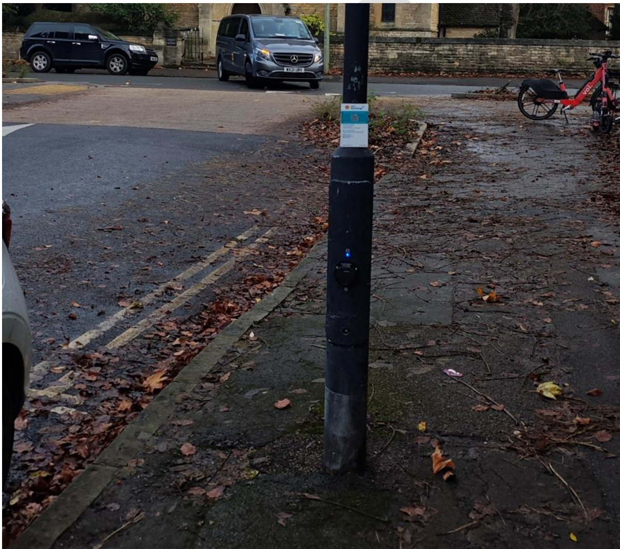
Figure 88: EV charging retrofitted into lamppost on corner of Leckford Road and Woodstock Road
