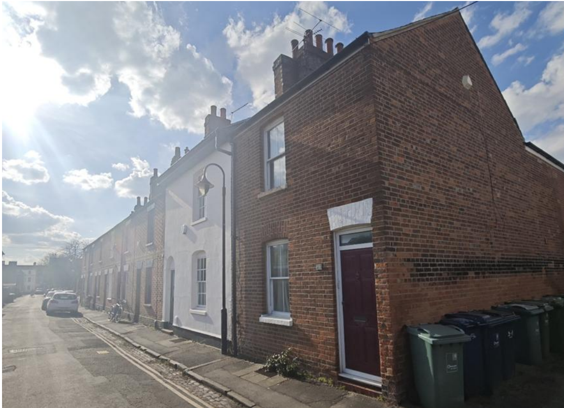
Figure 86: Introduction of render to traditionally exposed brick facades detracts from its character and appearance and can result in loss of architectural detail
