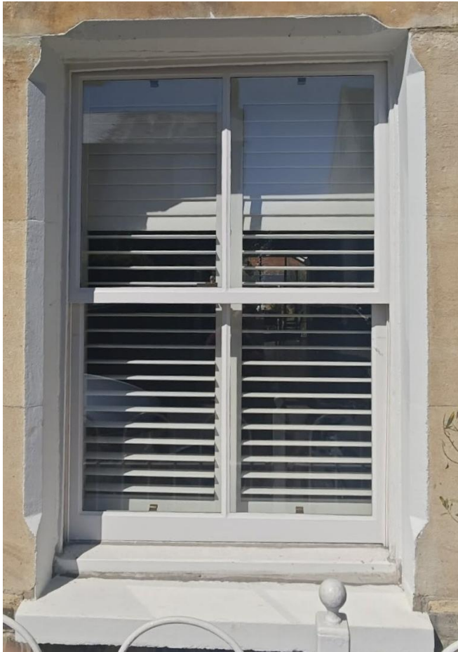
Figure 85: Original timber vs. Modern sympathetic replacement. Slimline double glazing in a traditional timber sash, proportional glazing bars with appropriate colour & detailing can improve the architectural character and appearance of a dwelling
